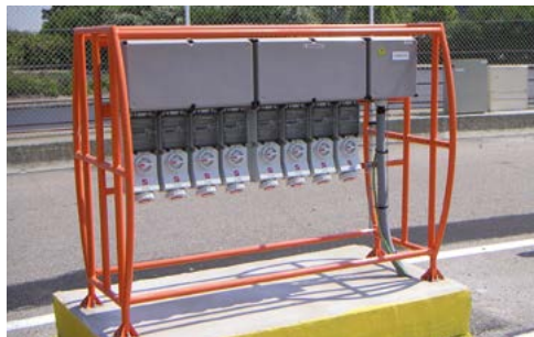
Container Terminal, Le Havre, France
