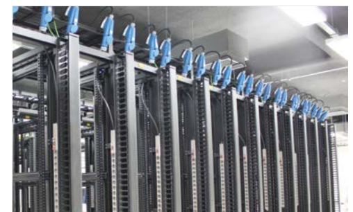
Internet Data Center, South Korea
